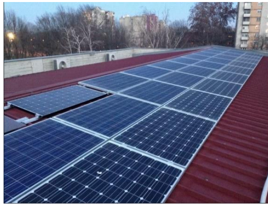
Figure 1. Installed PV modules on the roof in Osijek
